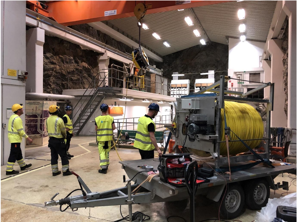
Figure 3. The Ocean Modules motor driven winch with 2000 meters of cable in the turbine hall.
